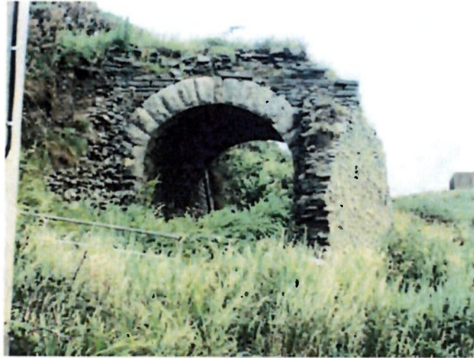
Photograph 11 Stone Bridge in Need of Urgent Repair
